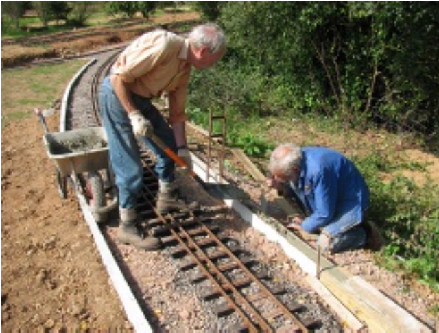
Photo 2: Ian Grinter and Mark Davis forming cast concrete edging along the track.
