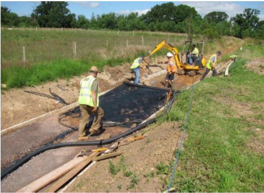
Photo 1: The steps in track construction are shown in this photo of the double track cutting. In the distance is the raw clay excavation, and nearest the camera is the finished trackbed ready for ballast laying.
